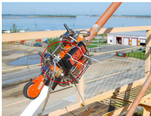
Figure 4. MRT of bridge rope. Data logger INTROS (circled) is fixed on magnetic head
